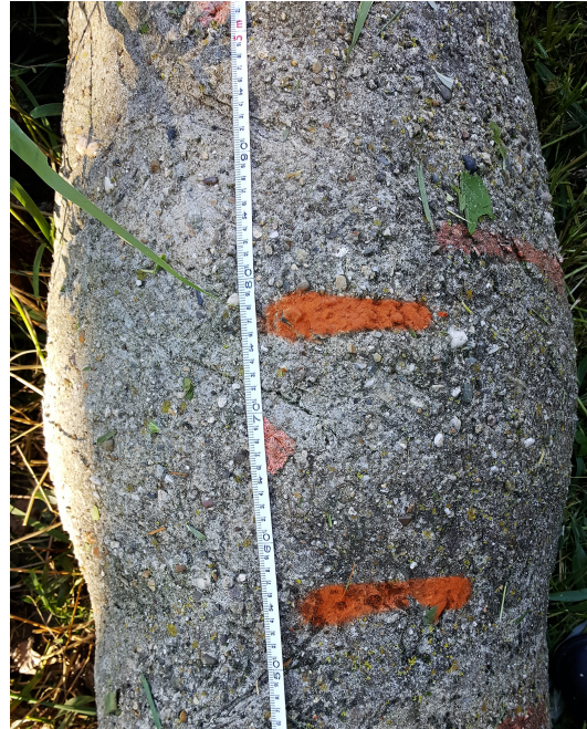
Figure 7-6: Photo of a bulge on pile 13 with part of a measuring tape.
