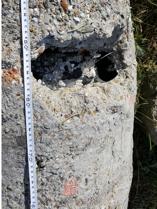
Figure 7-5: Photo of a created neck on pile 17 with part of a measuring tape.
