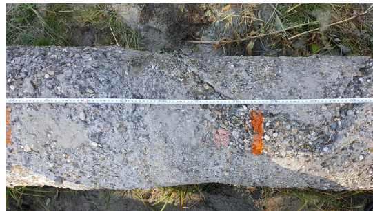
Figure A-2: Photos of diameter changes in pile 7.
