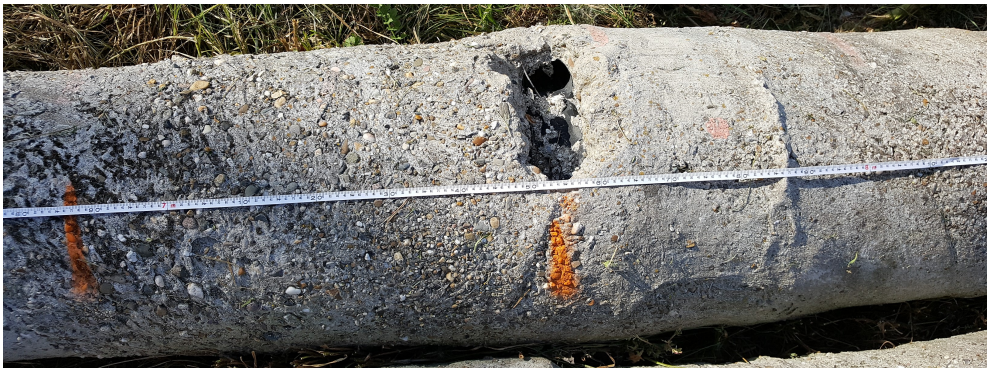
Figure A-5: Photo of a created neck on pile 17 and slight bulging with part of a measuring tape. Orange marks indicate the measurement location of the seismic tube.
