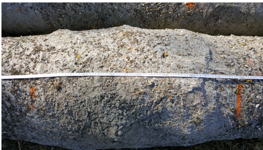
Figure A-1: Photos of diameter changes in pile 6.
