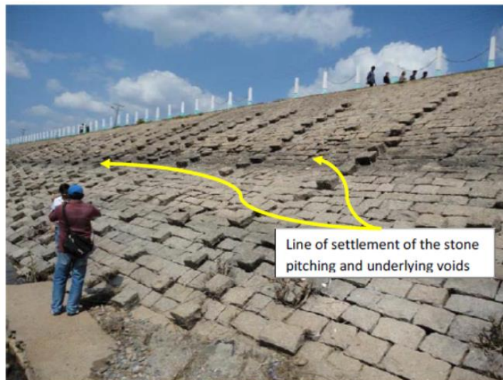
Figure 4.11. Settlements observed in upstream face of Saddle Dam 1. Source: Technical inspections.
