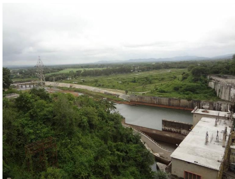
Figure 4.7. View of the right side protection wall of tail channel for left bank after completion of work. Source: CSV20170921.
