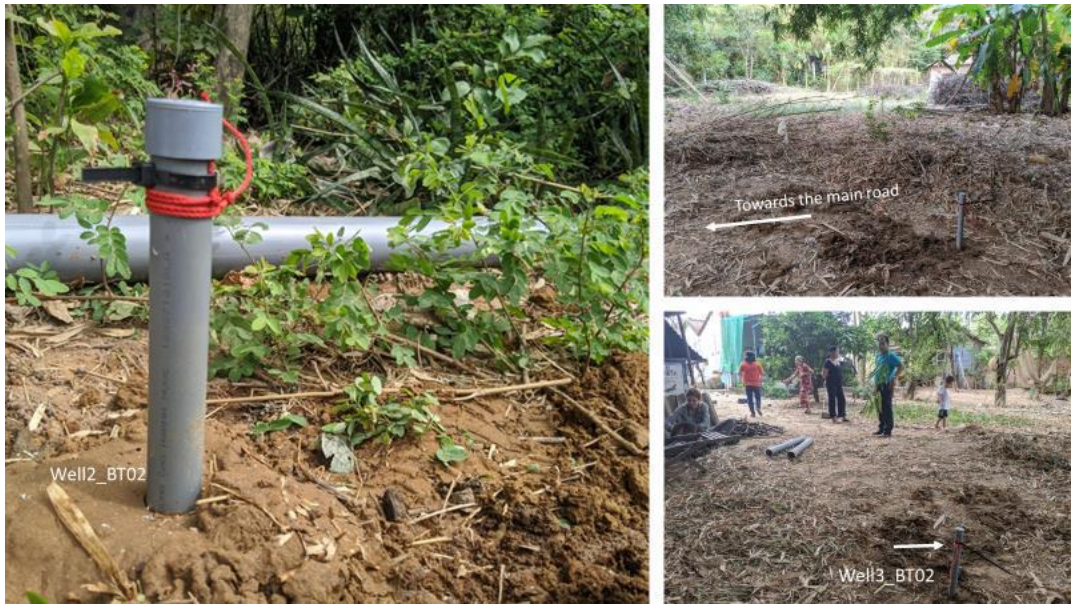
Figure 11-8: Well 2 and Well 3 at the BT2 site.
