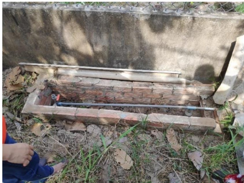
Figure 11-14: Example of a pump well (location 15).
