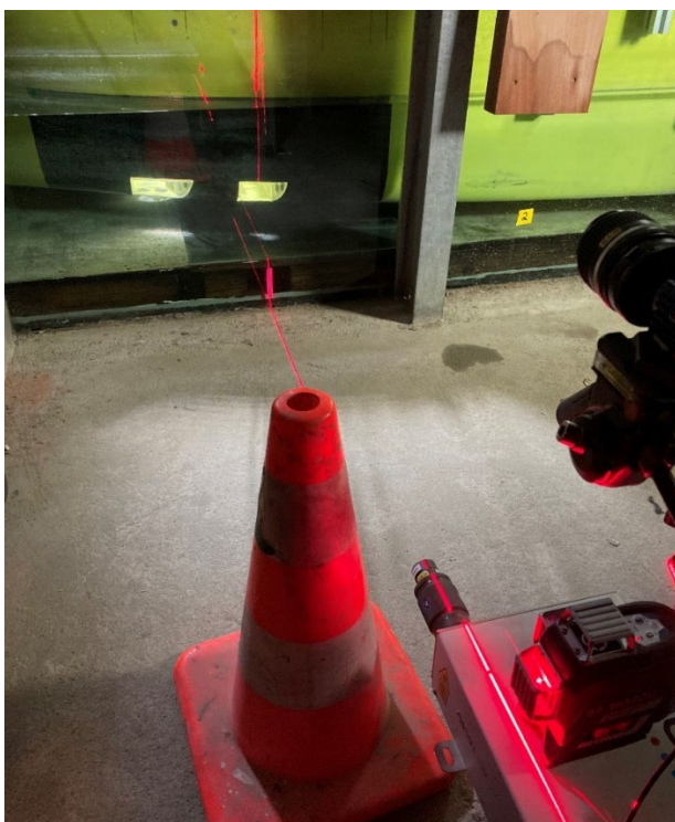
Figure 5.3 Cross-laser used to align the vessel in the y-direction..
