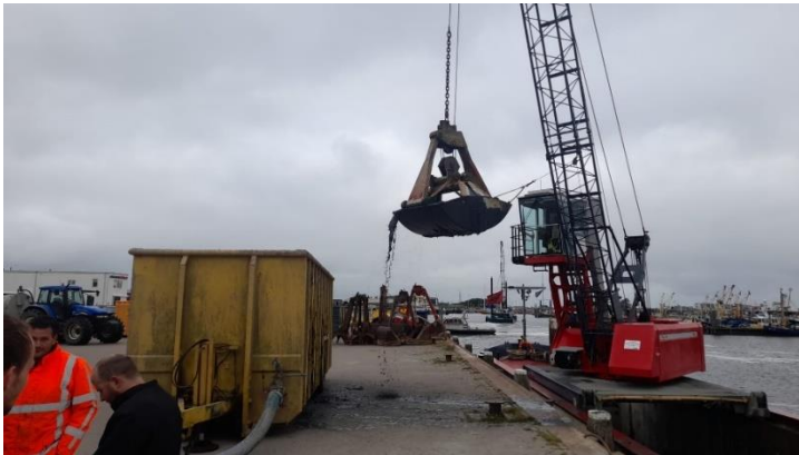
Figure 6.4: Unloading dredged sediment from the vessel using an excavator at the Lauwersoog harbour.
