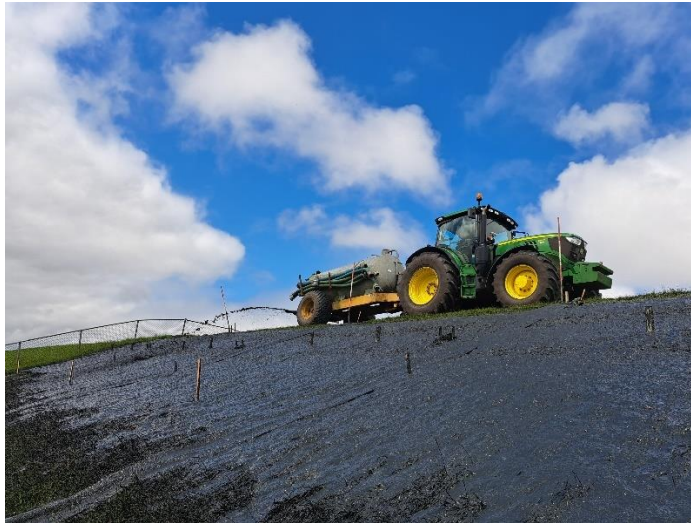
Figure 6.5: Application of the sediment from the top of the dike through a nozzle equipped on the slurry tank.
