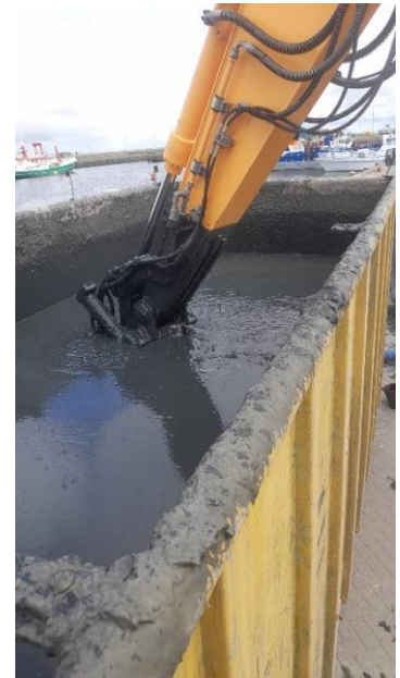
Figure 5.3: Mixing of the dredged sediment using a loader bucket equipped on construction tractor.
