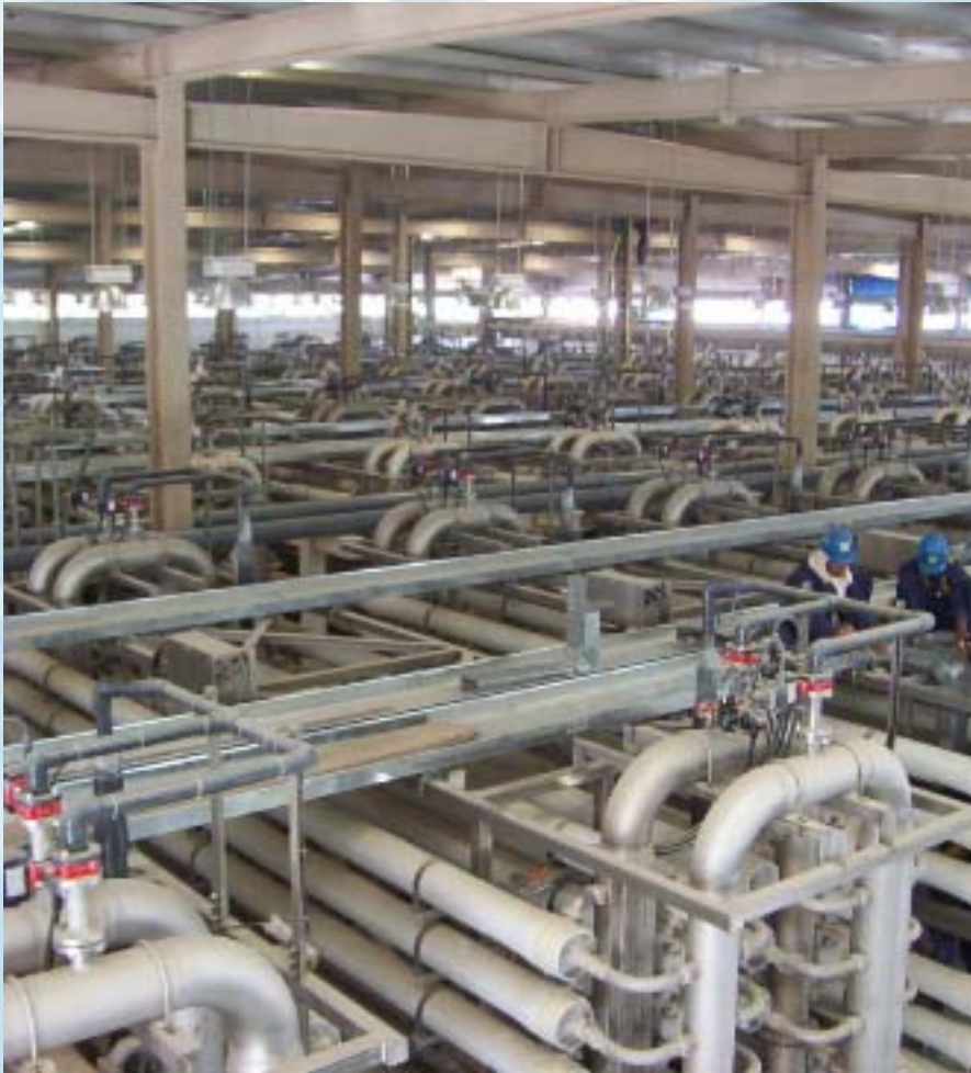
Sulaibiya UF-RO Plant (Courtesy of Ionics Italba S.p.A, Milano, Italy)
