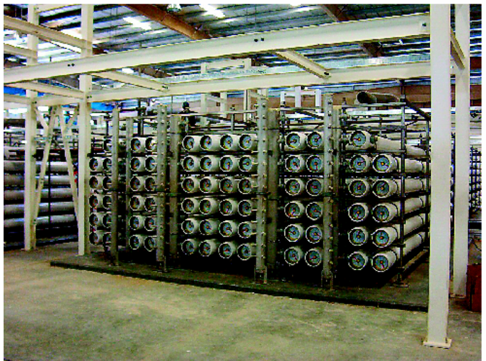
Reverse Osmosis vessels
