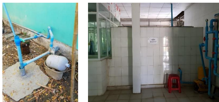
Figure 10a, b: the drinking water plant's private tube well (a, left). The storage (settling) tank (b, right).
