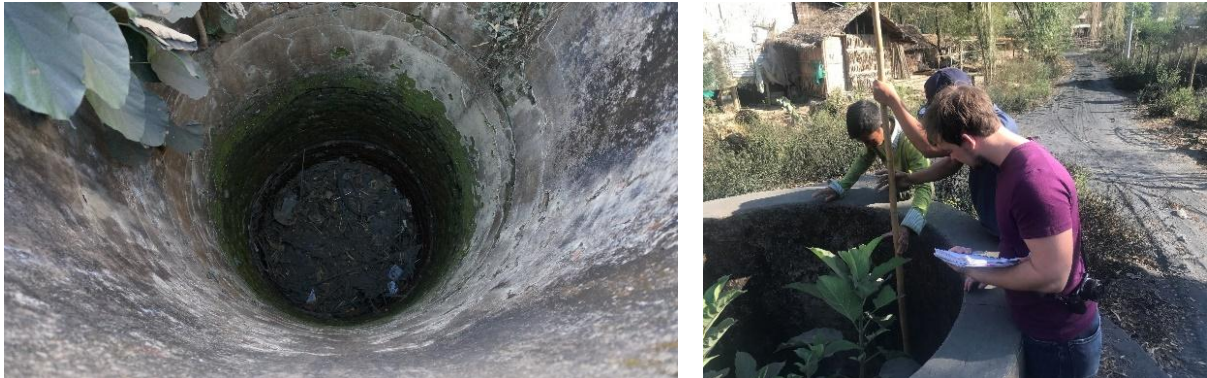
Figure 17a, b: the well appears to be dry (a, left). Measuring the well depth with a stick used for drying clothes (b, right).
