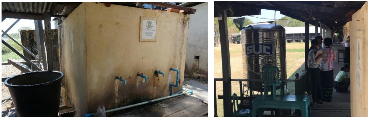
Figure 7a, b: settling tank donated by Japan (a, left). Rain water collector (b, right).
