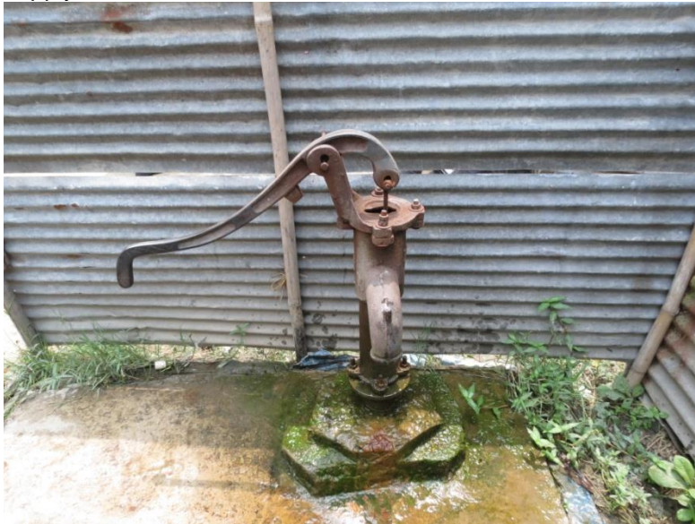
Figure 8: Typical tube well for domestic water supply in Bangladesh.
